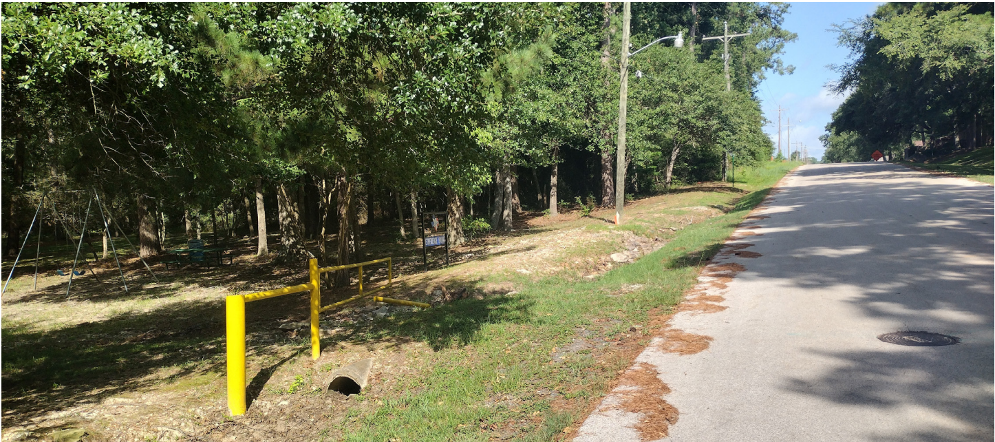
The open ditch and lack of sidewalks creates access issues at Emma Etheridge Park.
