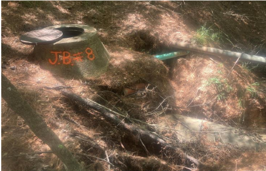
MH #8 near Back Common Corner of 1652 and 1656 Green Briar Dr. 18" near property line, with 10' Utility Easement. Other Utilities Lines near it.
