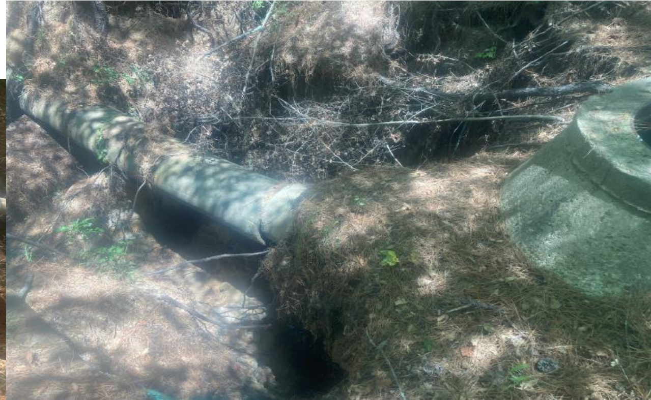
Storm Water Breach in Line due to Severe Erosion, And Lack of Vertical Support.
